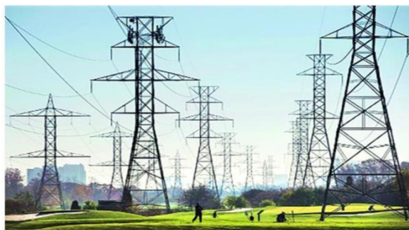
Fig no.1: Transmission Tower
